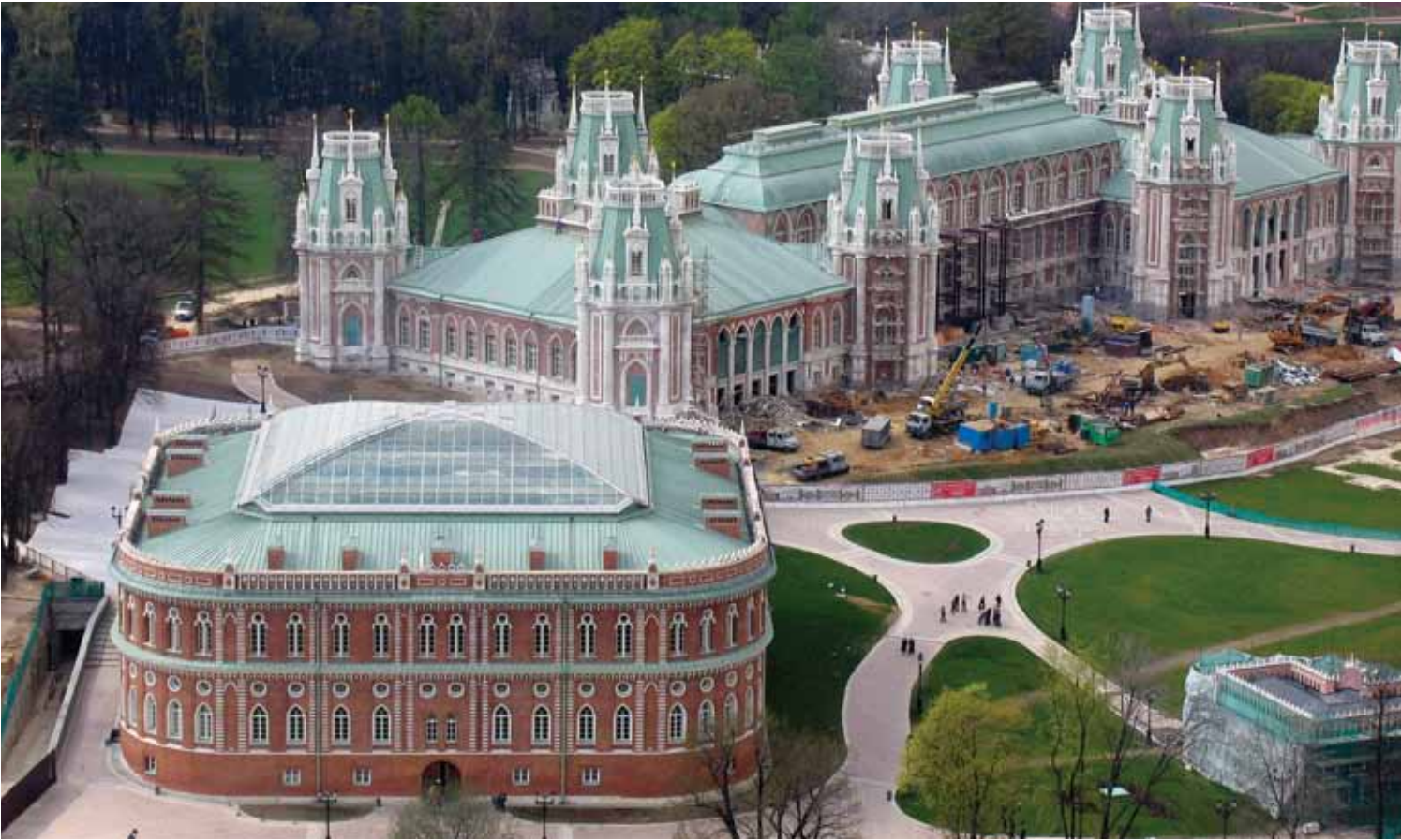
Large areas of Long Strip roofing, created with Nordic Green™ pre-patinated copper, are used throughout the Tsaritsyno Palace in Moscow.
